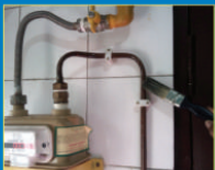
PNG PIPE LINE
