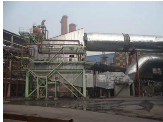
Sinter Cooler Waste Heat Recovery Equipment (Wuhan Steel in China)
