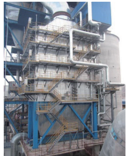
PH Boiler First Machine (Huaibei Cement in China)
