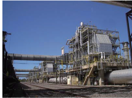
Waste heat recovery power plant for coke oven (SOL CST in Brazil)
