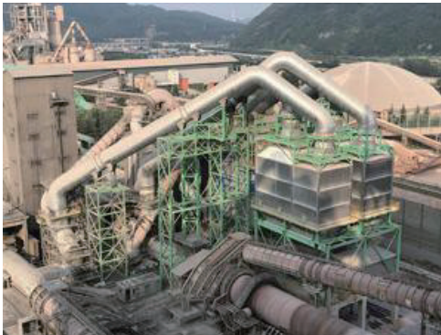
Cement Waste Heat Power Generation Equipment (Ssangyong Cement South Korea Donghae plant)
