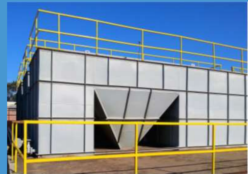
SEWAG TREATMENT PLANT (TRICKLING FILTER/SAFF)
