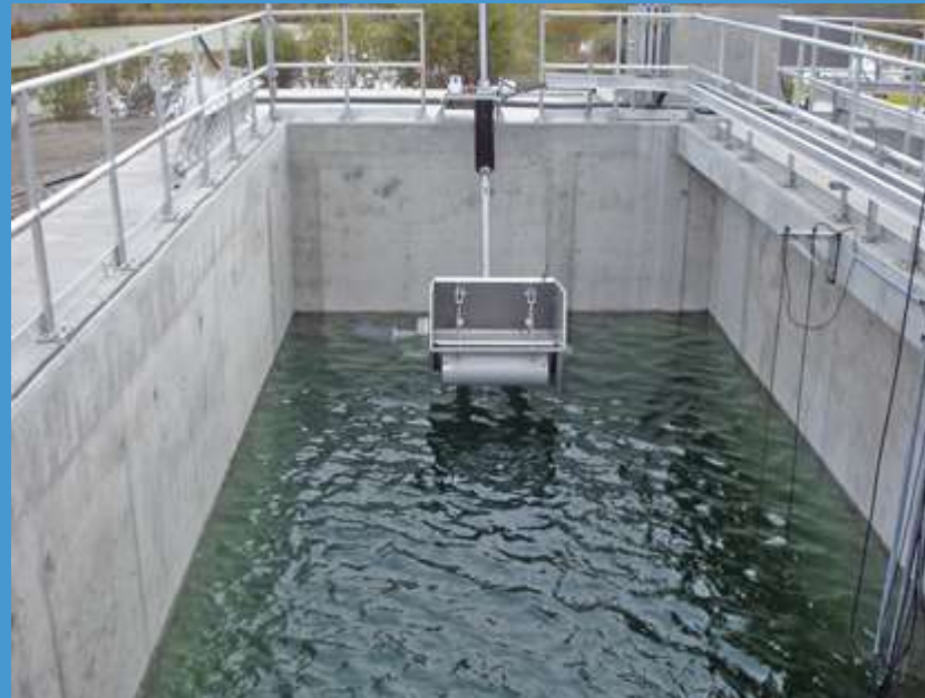
SEWAG TREATMENT PLANT (SBR)
