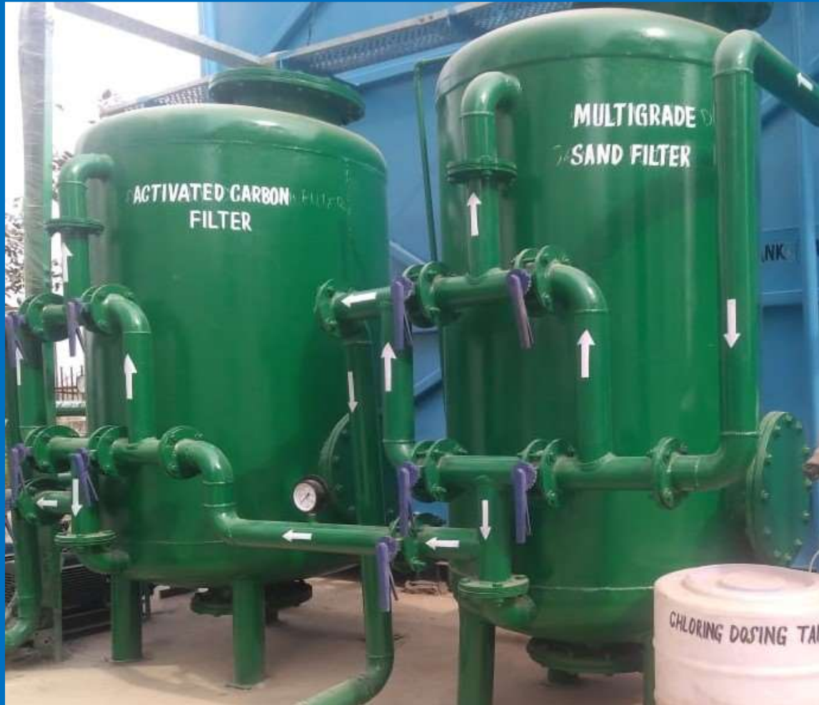
MULTI GRADE FILTER & ACTIVATED CARBON FILTER (MGF, DMF, SAF & ACF)
